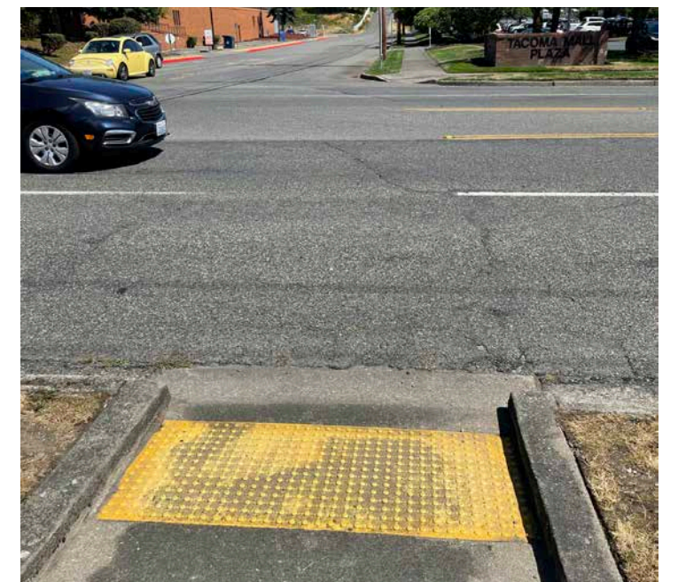
Unmarked crosswalks at S 42 nd St
