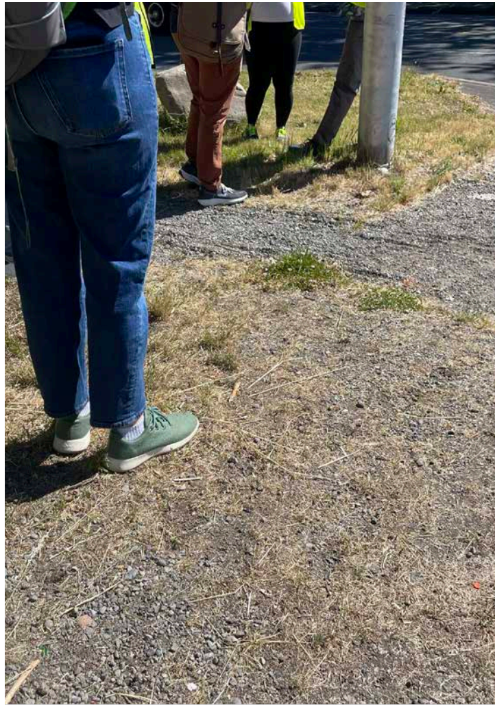
Dirt and gravel covering sidewalk at northwest corner near S 21st St
