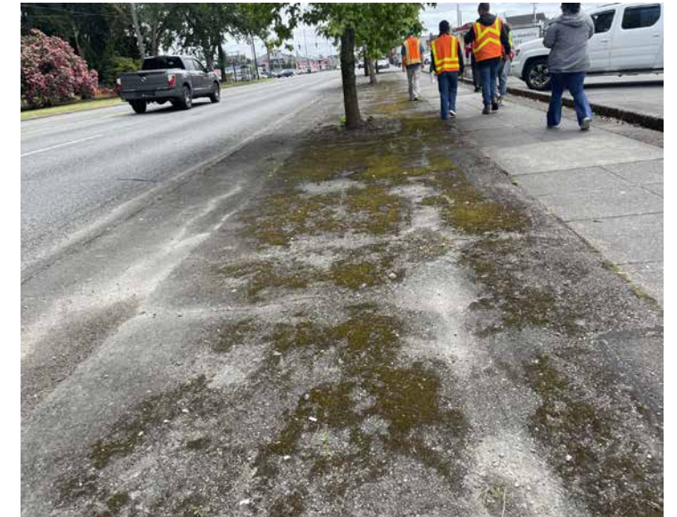
West side of street needs depaving between S 47 th and S 50 th St
