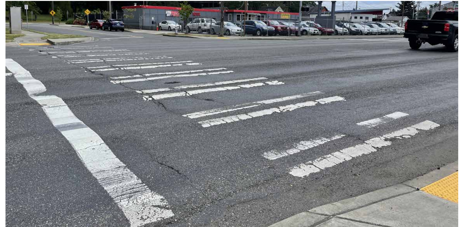
Concaved roadway in need of improvement
