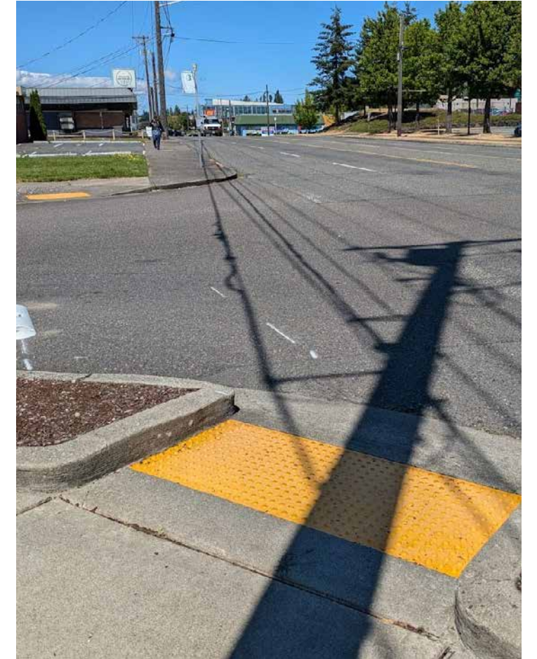
Curb ramps misaligned at S 40 th St
